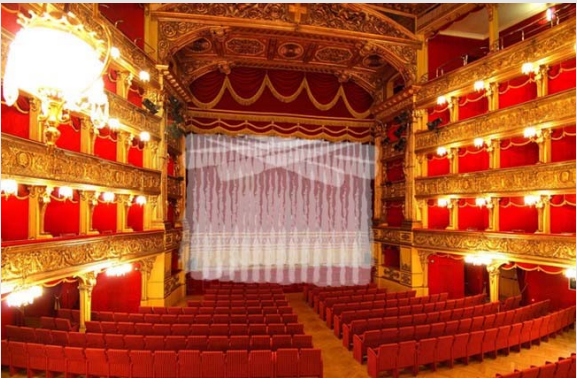
Test of a water mist curtain Spraytecs for the protection of a theater curtain and the surrounding décor.
